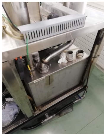
Figure 21 Dedicated tank for the scrubbers water (containing water+ ice)
