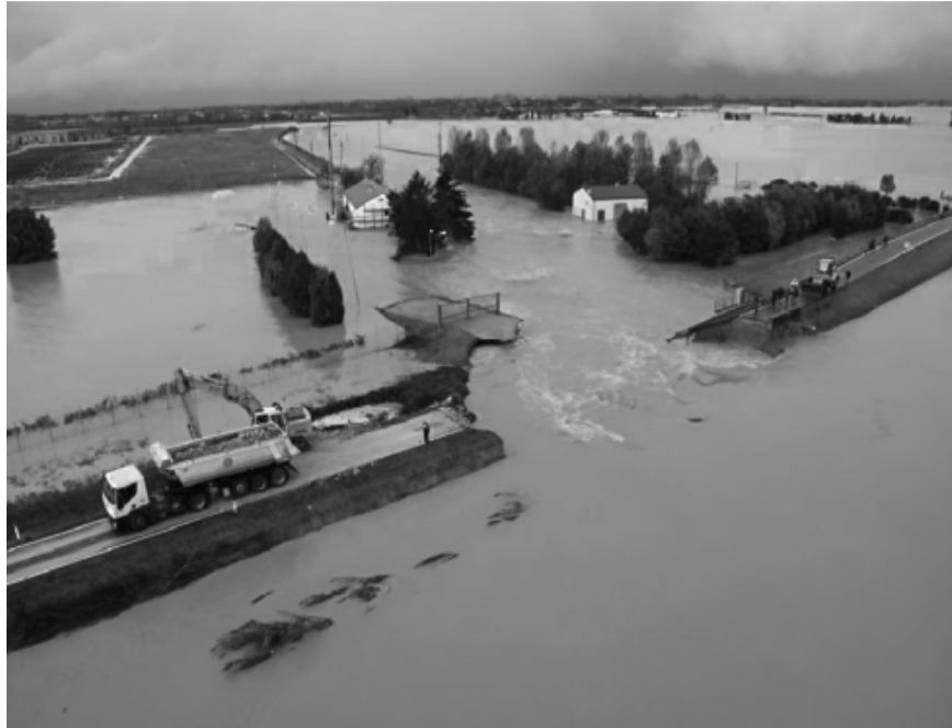
Breach of the Bacchiglione-Roncaiette embankment near Ponte San Nicolò (PD)- Flood of 2010 Source: Compagno, 2019
