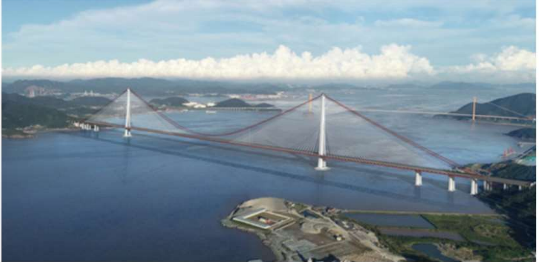
Construction of the Xihoumen railway-highway dual-use bridge, a key project of the Ningbo-Zhoushan Railway, is ongoing in Zhoushan, East China's Zhejiang Province on August 6, 2023. (Photo/Screenshot from website)
